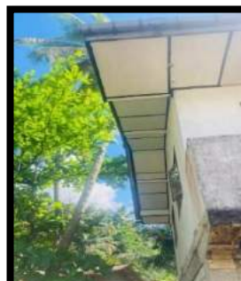
Repairing the roof of the multipurpose building near the Ayagama weekly fair Ayagama Pradeshiya Sabha – Sabaragamuwa Province Expenditure - Rs.
