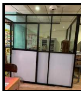
Fixing a front roof for the Baddegama Public Library Baddegama Pradeshiya Sabha – Southern Province Expenditure - Rs. 250 000 00
